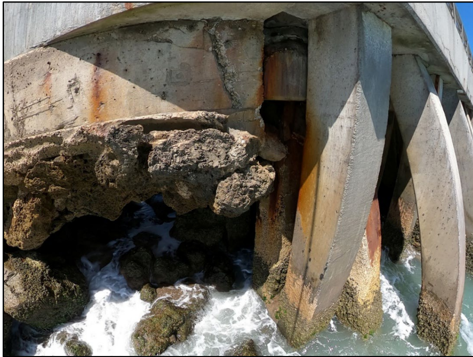
Figure 1 – Armor/Crib Stone Erosion and Settlement at Phase 2-3 Transition
